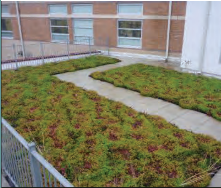
Vegetative roof during a wet weather event in October 2011
