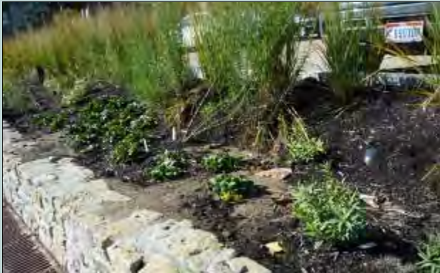
Sand washed out of the amended soil above the topsoil.
