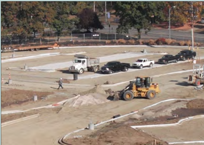
Stock piled raw materials adjacent to the porous pavement areas under construction, vehicles parked on features.
