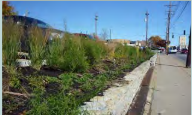
Bioswale overview illustrating sand washout onto adjacent wall.
