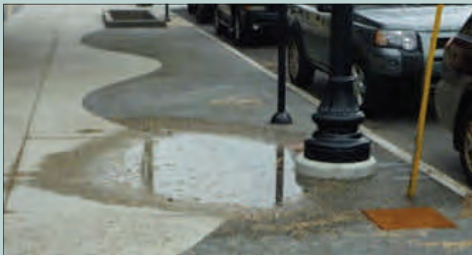
Stormwater ponded on the porous concrete sidewalk.
