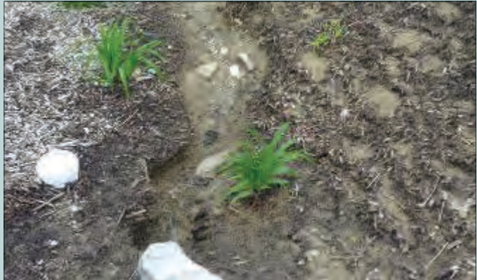
Erosion in the bioinfiltration basin.
