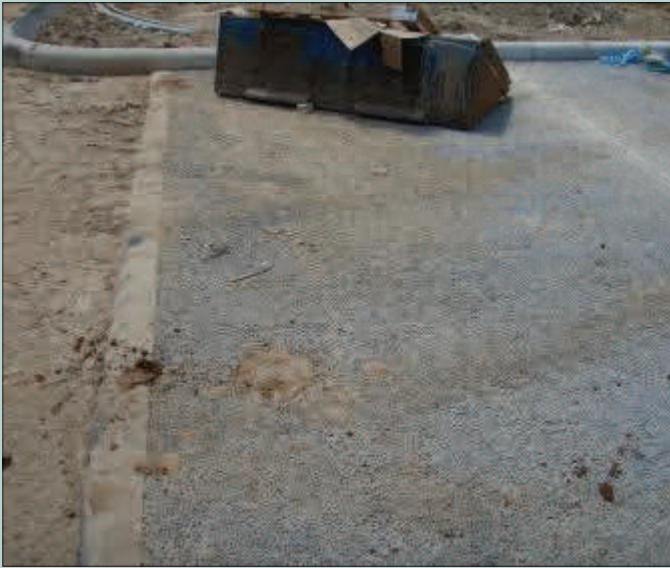
Exposed dirt adjacent to the newly installed porous concrete can cause sediment build up and clog the system.
