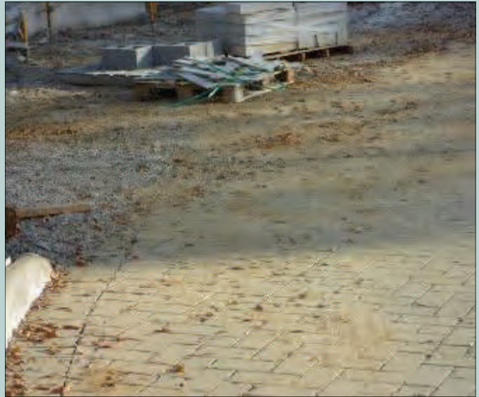
Exposed dirt adjacent to the newly installed porous paver system can cause sediment build up and clog the system.
