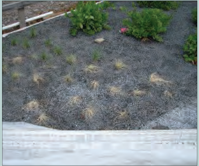
Dead plants on the vegetative roof.
