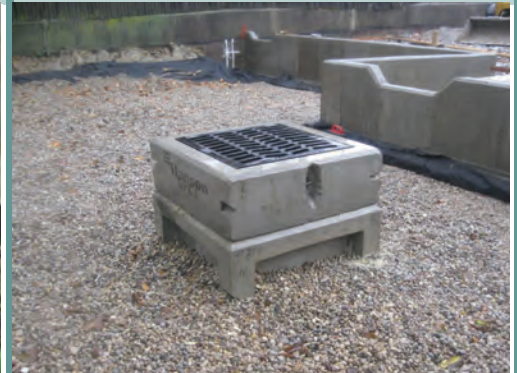
Bioinfiltration Facility with Overflow Structure
