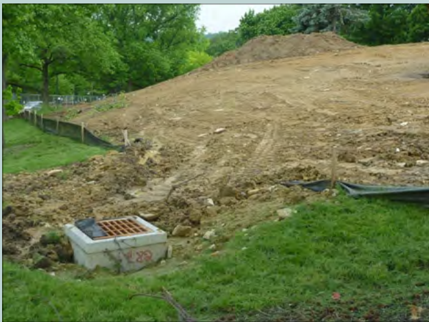
Broken silt fence promotes erosion and sediment build up in the proposed green feature.
