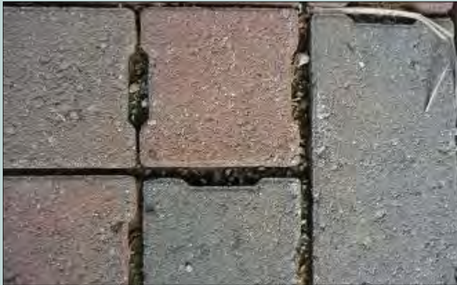
Sediment built up in the porous paver system.
